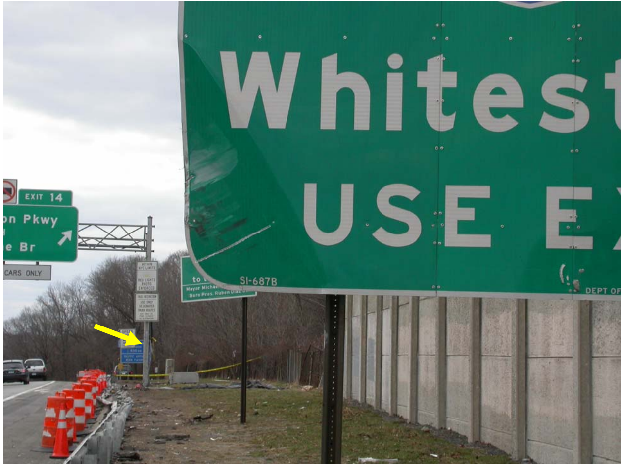
Figure 6 - Close up of contact damage from the bus found on the first sign shown in figure 5. The main damage to the second sign was to the left side support post which was destroyed by the impact with the bus. Arrow in the background highlights the overhead sign stanchion which the bus struck before coming to final rest. Note damage to guardrail just before the overhead sign stanchion. This damage suggests the bus was rolled approximately 90 degrees to the right at this point.
