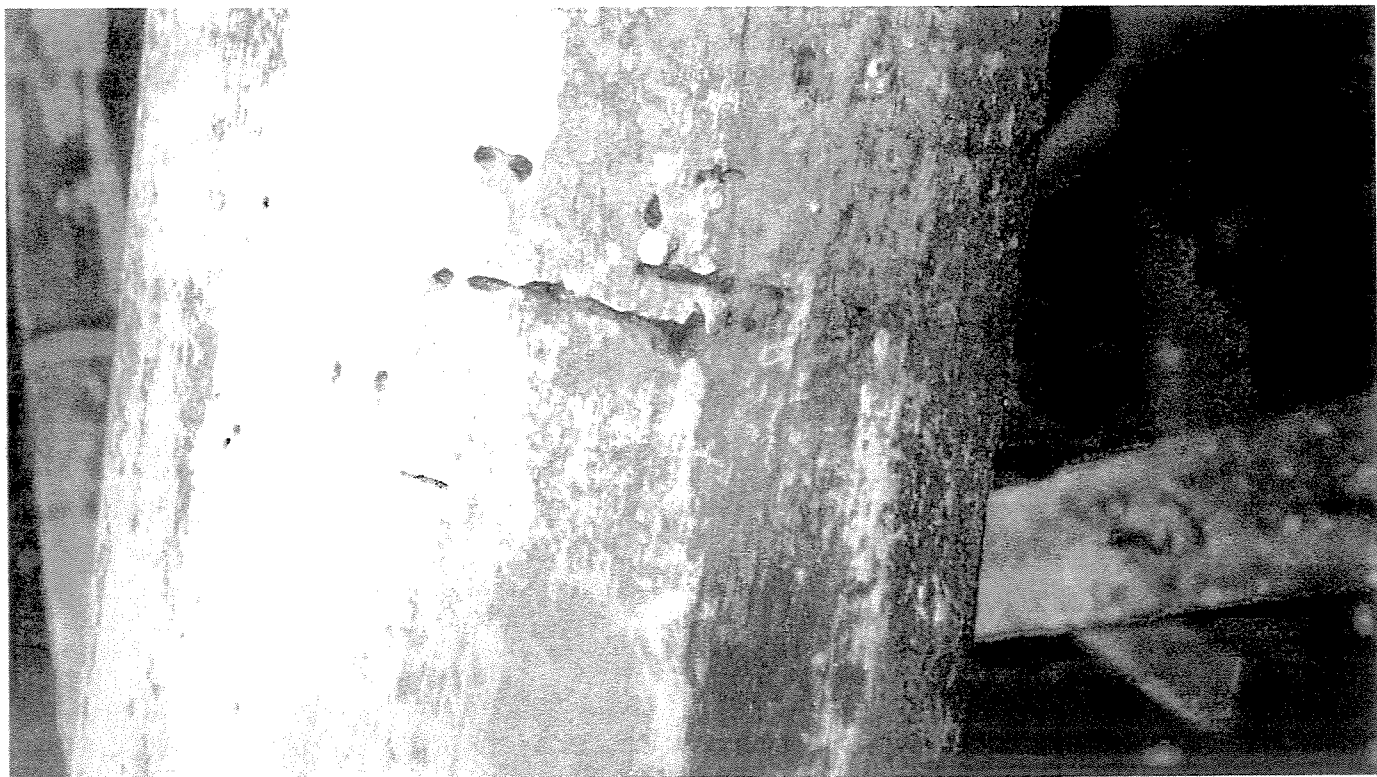
PHOTO 10 – Pile 61 I (batter). Moderate localized Teredo marine borer activity on outer annulus of the greenheart pile, looking NW.
