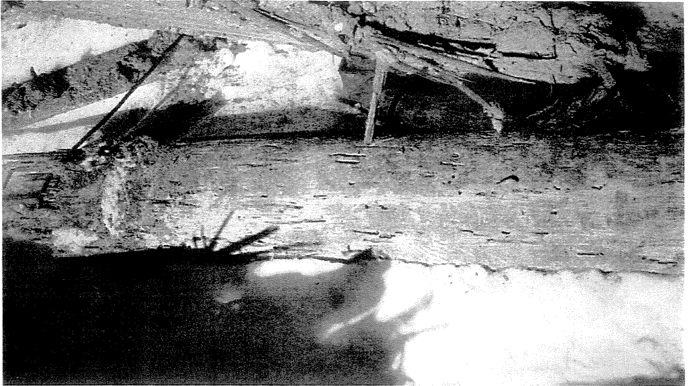
PHOTO 13 - Greenheart pile on top of the deck ("pulled" from the mud). Typical of view of moderate Teredo activity observed below water at various greenheart piles from mean-low-water to the mudline.
