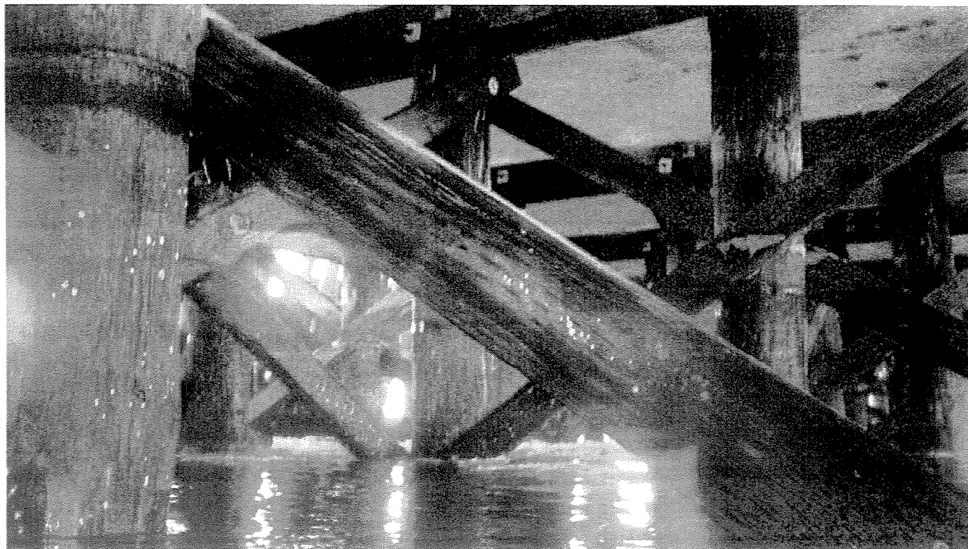
PHOTO 2 – Bent 66 between piles "E" and "F." Brace exhibits rot in the tidal zone with 50% loss of cross-sectional area looking east.
