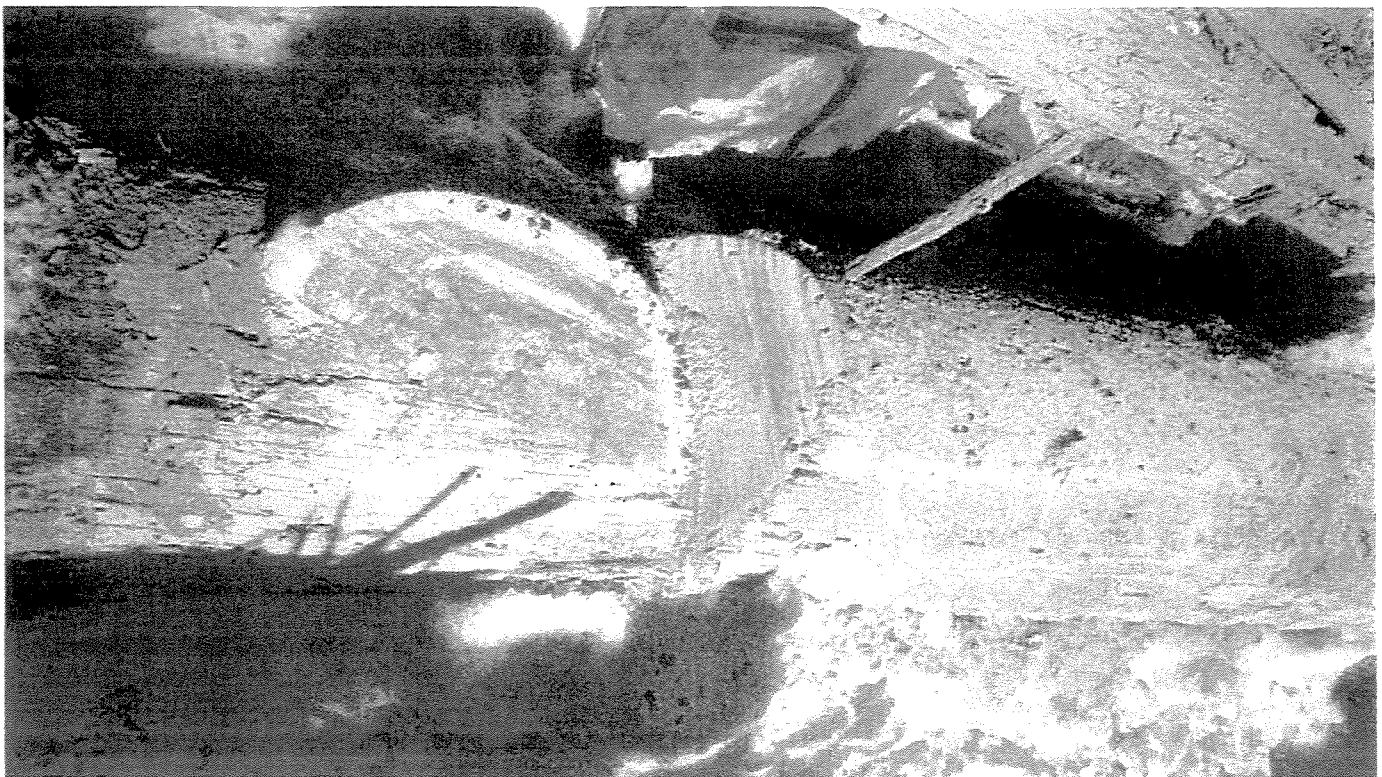
PHOTO 14 - The above referenced pile was sectioned with a saw revealing a solid inner core. Damage is limited to the outer annuls with no significant loss of cross-sectional area.
