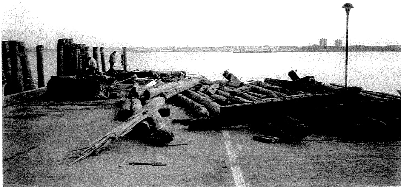
PHOTO 7 - Top side view with pulled fender system piles on top of the pier, looking east.
