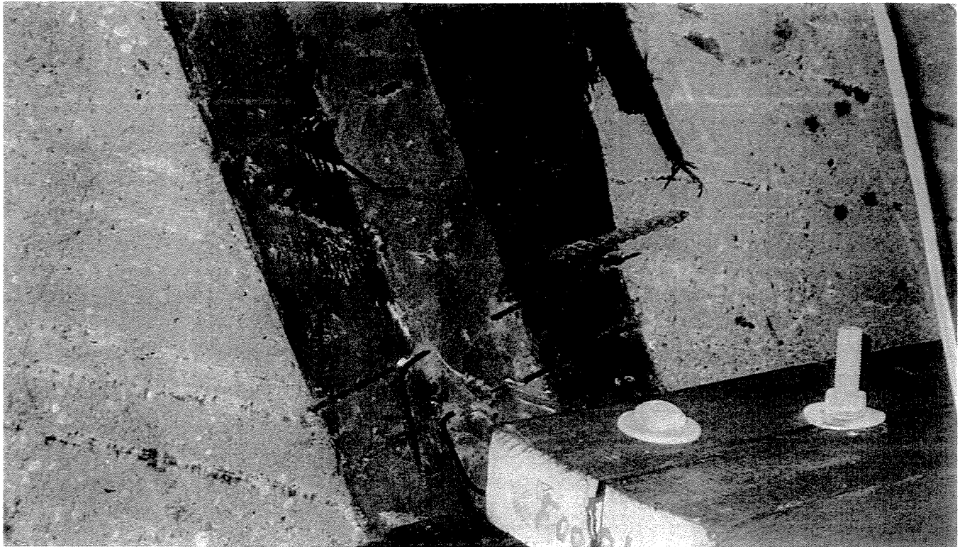
PHOTO 13 - Pile bent 78, close-up of collapsed deck showing 1/4" diameter steel "ties," sets of four (4) at 12" spacing. Steel ties assumed to have provided connection between concrete deck and timber pile cap, looking south.
