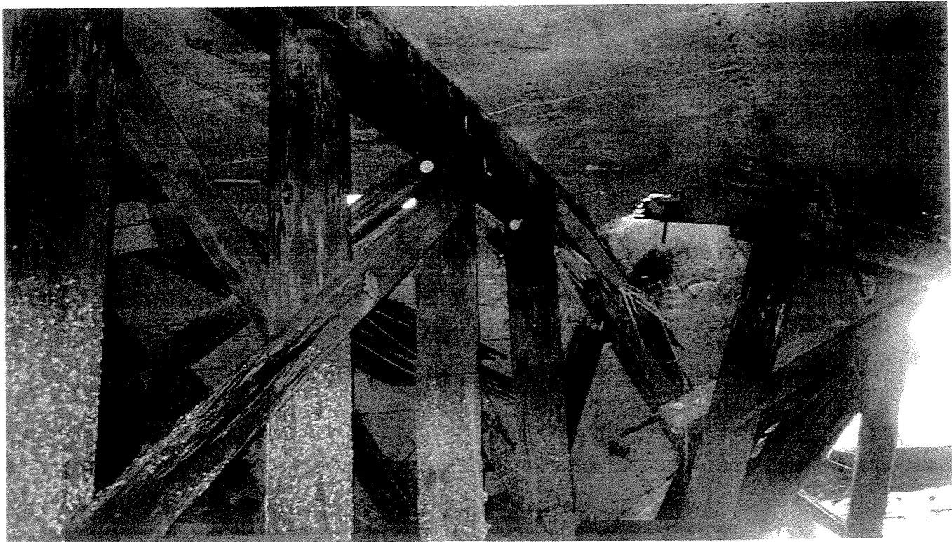
PHOTO 14 - Pile bent 77, general view of impact damaged, collapsed underside of pier. Piles "D" thru "I," timber cap beam broken south of "G" pile with severe displacement of "H" and "T" piles, looking SE.
