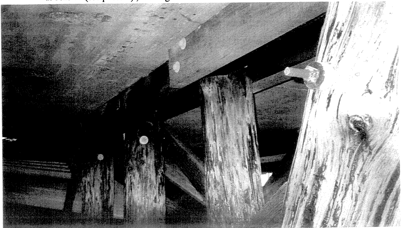
PHOTO 10 – Bent 78, piles "A-batter," to "D." Bent numbers 78 and lower have a dual 6 x 12 timber cap with a "sistered" 6 x12 from piles "B" to "A" and "H" to "I" providing a 2' long cantilever on the outside perimeter of the pier for support of the concrete deck above, looking SW. Refer to section.
