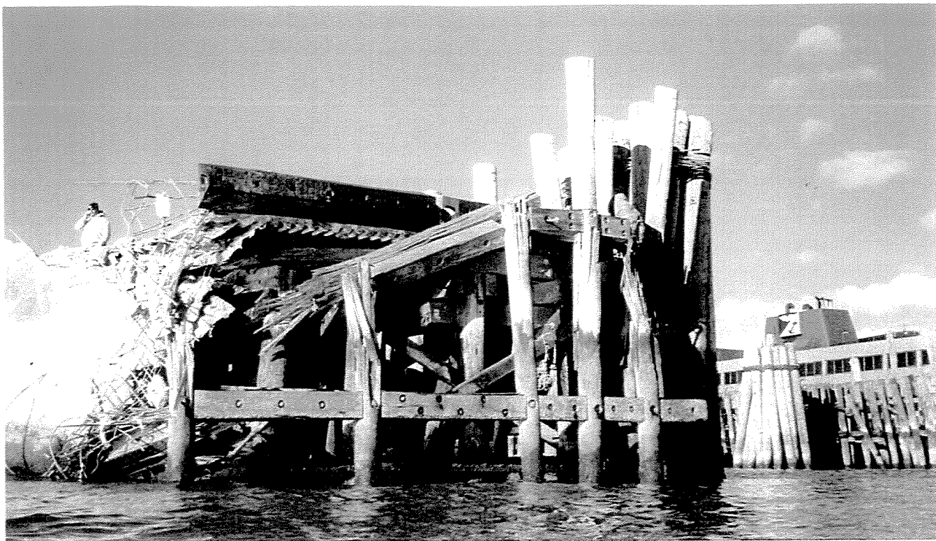
PHOTO 3 - East end of pier, approximately 20' along the east face remains erect at north end.
