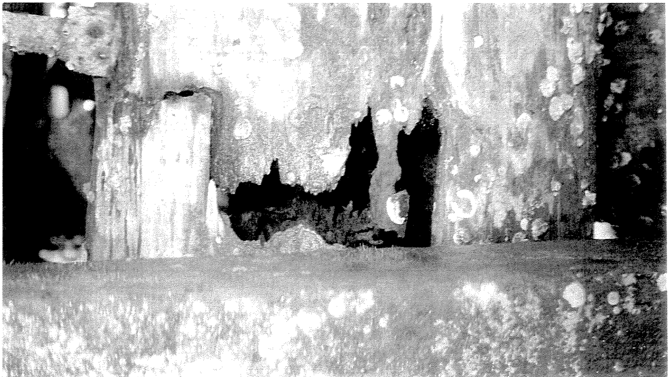
PHOTO 20 - Bent 80, "B" pile, close-up view of hole in pile, 2" above the lower horizontal brace. Note, pile exhibits hollowing with 95% loss of cross-sectional area and heavy marine borer activity.
