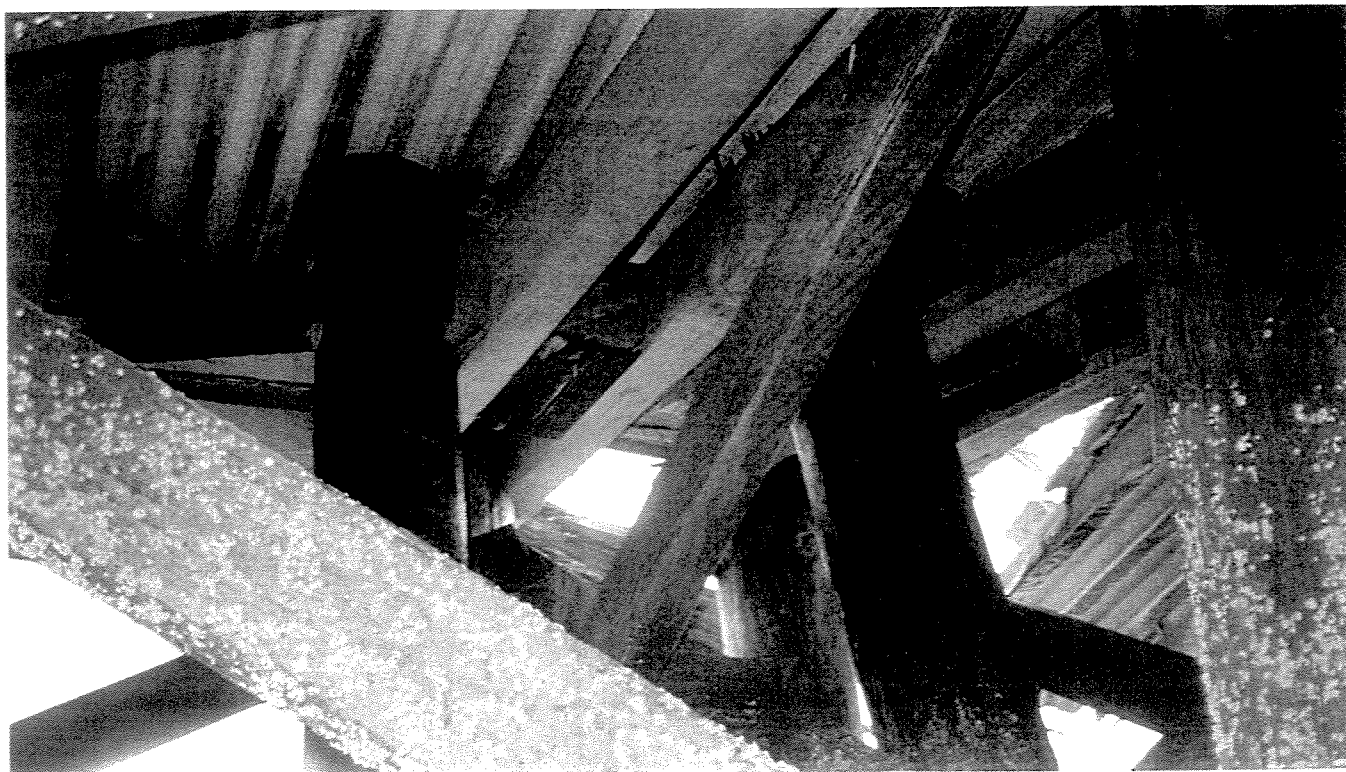
PHOTO 8 - Bent 80, piles "C" and "D" with "C-batter" and "D-batter" showing general configuration and construction. Note, top horizontal 6 x 12 bracing provides connection of battered piles to bent 80 and 79 vertical pile, looking SE.
