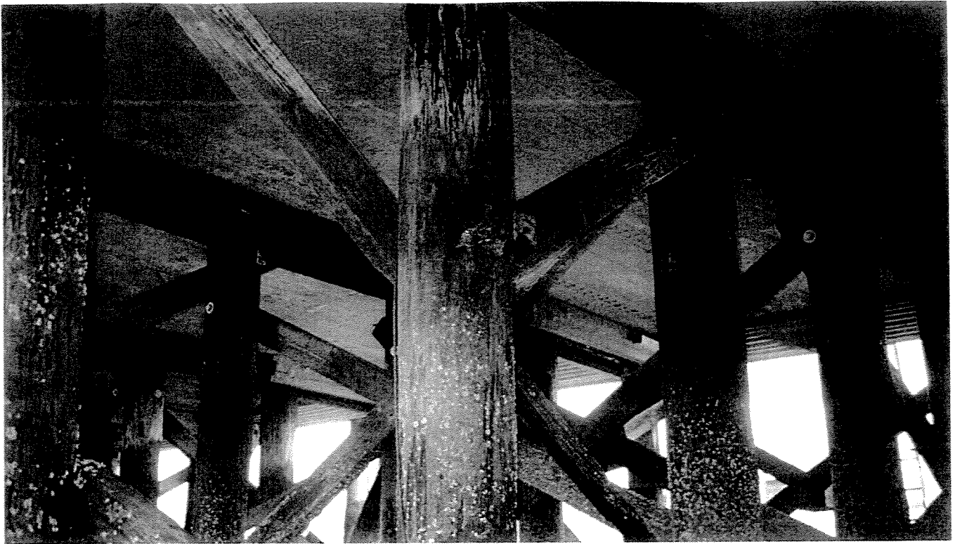
PHOTO 19 - Bent 76, "E" pile, diagonal 4 x 8 timber brace broken. Deficiency does not appear to be the result of impact damage.
