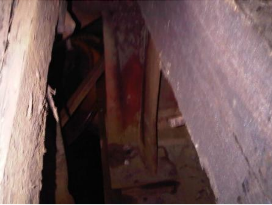
Photo B6. NW bearing stiffener, E girder, Span 3
