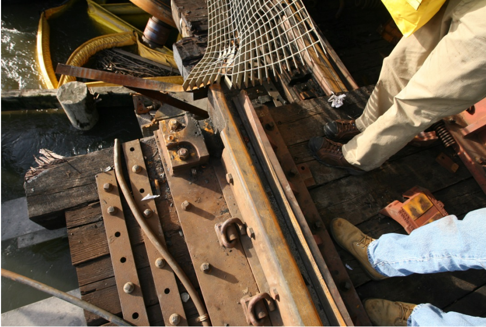
Figure 1A Northeast Slide Lock Assembly on the North Approach Span and POD
