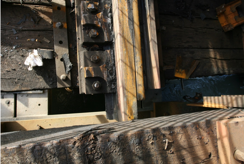
Figure 3A Northeast Slide Lock Assembly on the North End of the Swing Span and Initial Sign of Wheel Marks Crossing the Movable Bridge
