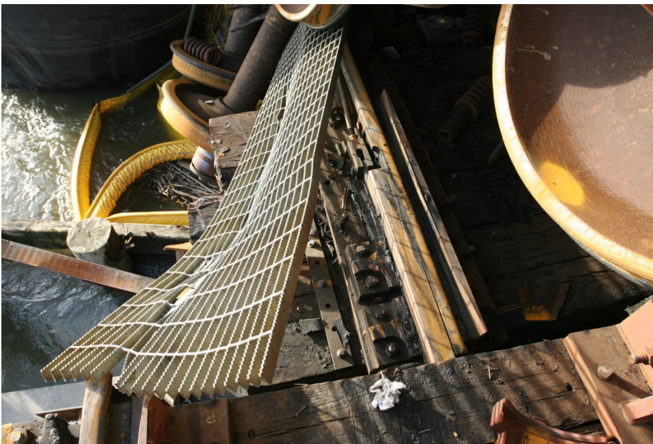
Figure 2A Northeast Slide Lock Assembly on the North Swing Span and POD
