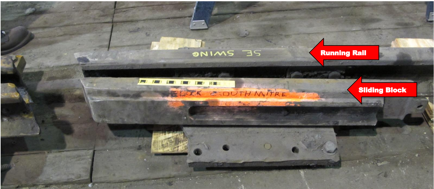
Figure 8. View of the south side east rail lock showing extensive damage to the bridge side components including; separation of the guide rail section with fracturing of the attaching bolts and release of the sliding block. View looking west.
