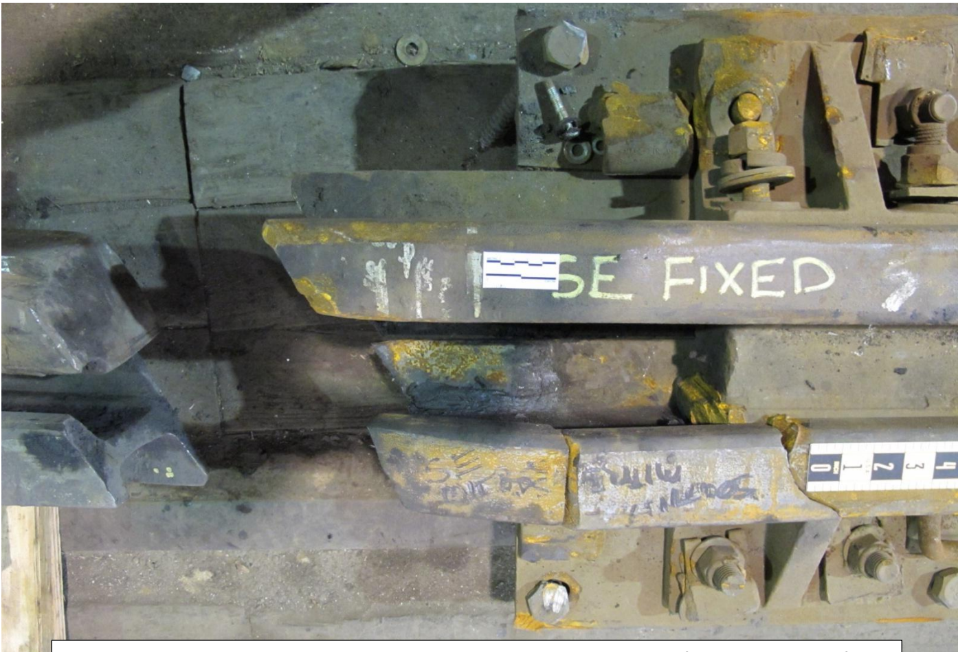
Figure 9. Upper view shows a side view looking east at the fractures in the fixed east running rail, south side adjacent to the gap. Lower view shows the same fractures from above relative to the grease line in the locking slot.
