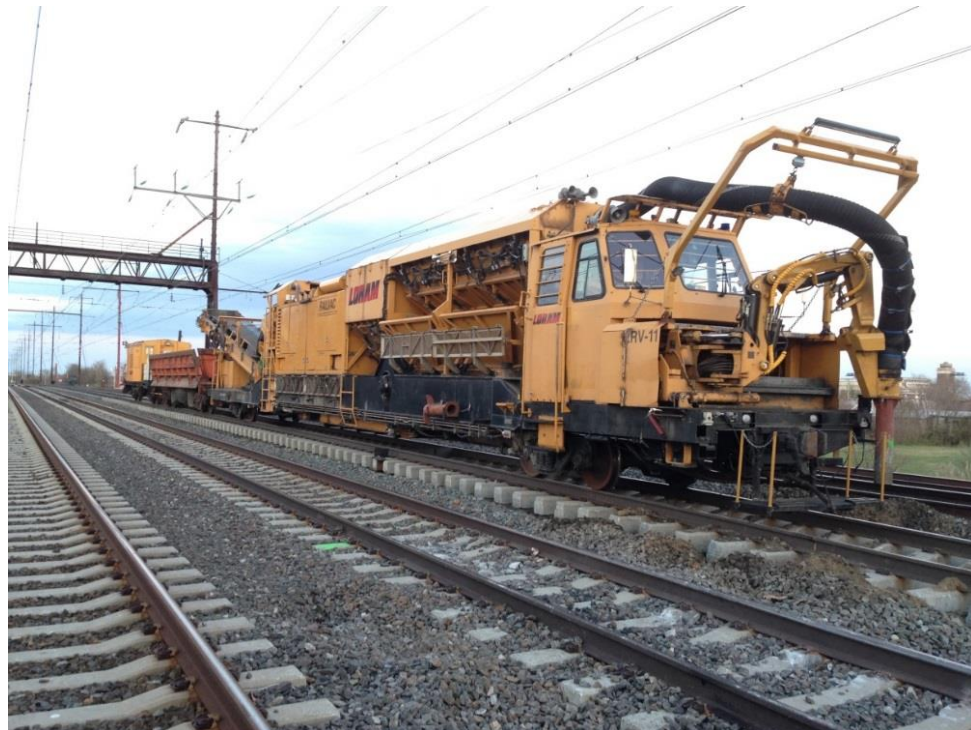
Figure 4. A view looking northeast at the Loram vacuum train as found on main track No. 2.
