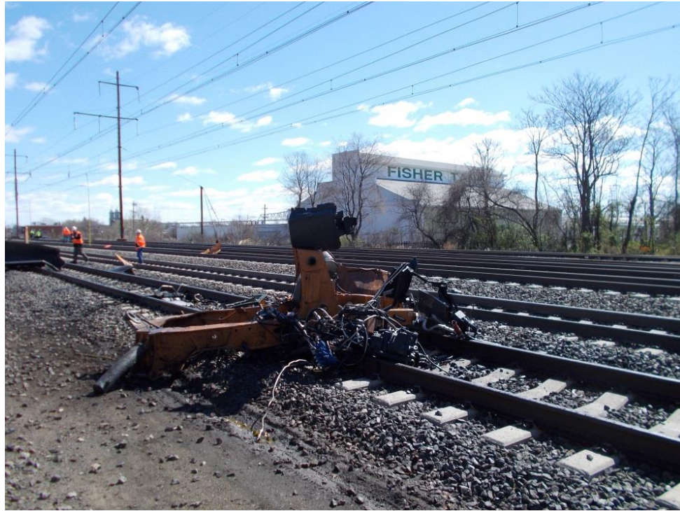
Figure 3. This is a view of debris as found on main track No. 4.
