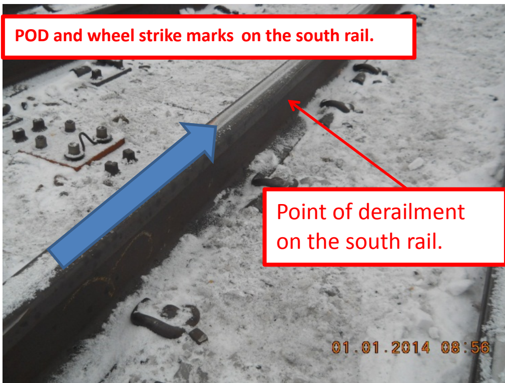
Figure 4. View of south rail derailment marks; blue arrow indicates direction of train travel.
