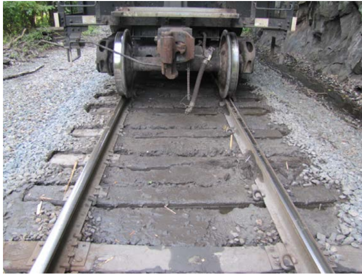
Figure No. 8. View of a fouled ballast condition Preceding the derailment footprint.
