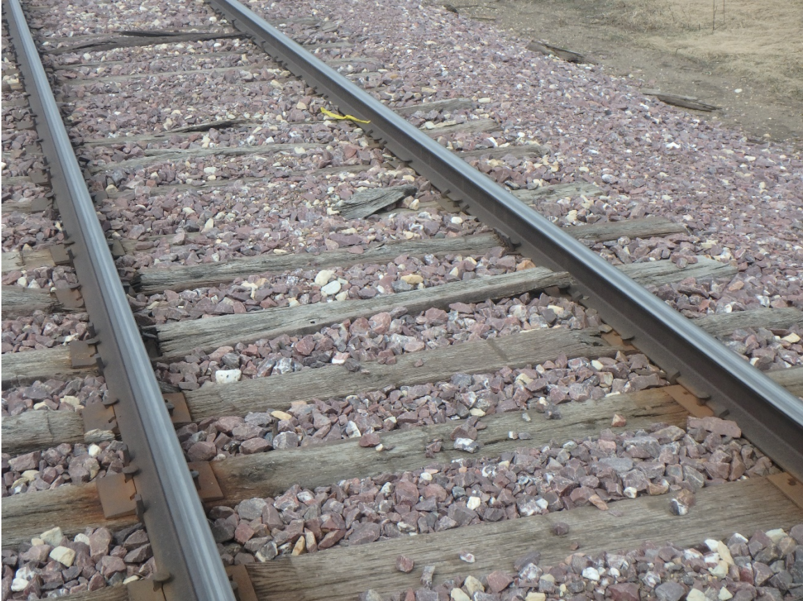
Figure 7. Split, broken cross-ties not holding fasteners in the track west of the accident area near MP 56.9. (NTSB Photo)
