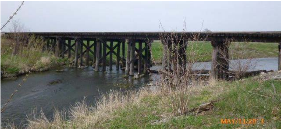
Figure 3. Bridge 56.72, spanning Jack Creek. View of the open deck bridge substructure (UP Historical Photo)
