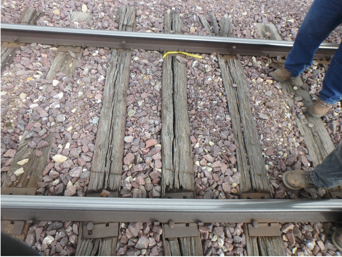
Figure 6. Split, broken cross-ties not holding fasteners in the track immediately west of the accident area near MP 56.9. (NTSB Photo)
