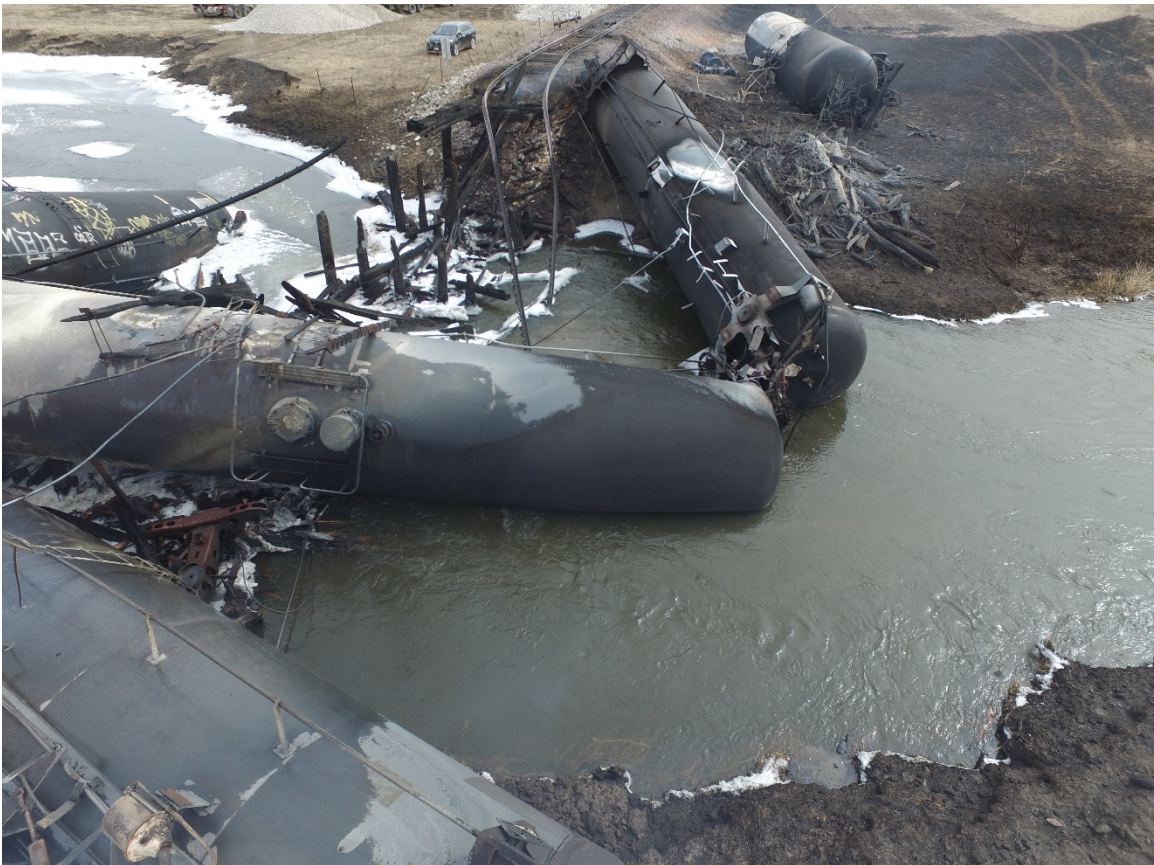
Figure 4. Jack Creek bridge destroyed as a result of the derailment and ensuing fire.
