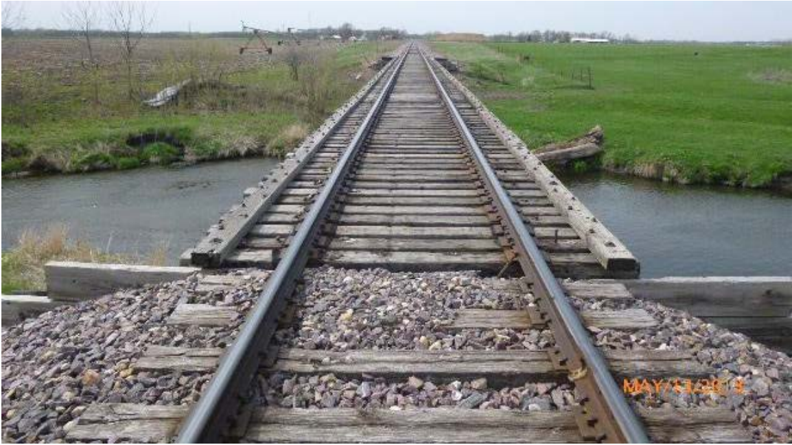
Figure 2. Bridge 56.72, spanning Jack Creek. Photo shows the bridge deck of the open deck bridge (UP Historical Photo)
