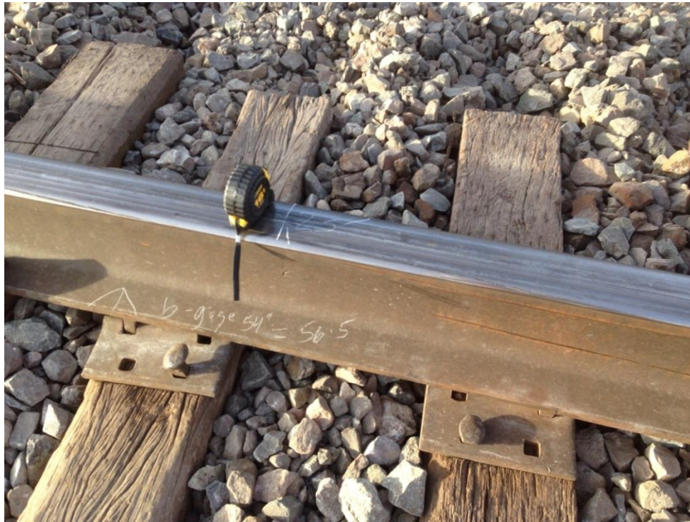
Figure 7. This is a view of the point of derailment.
