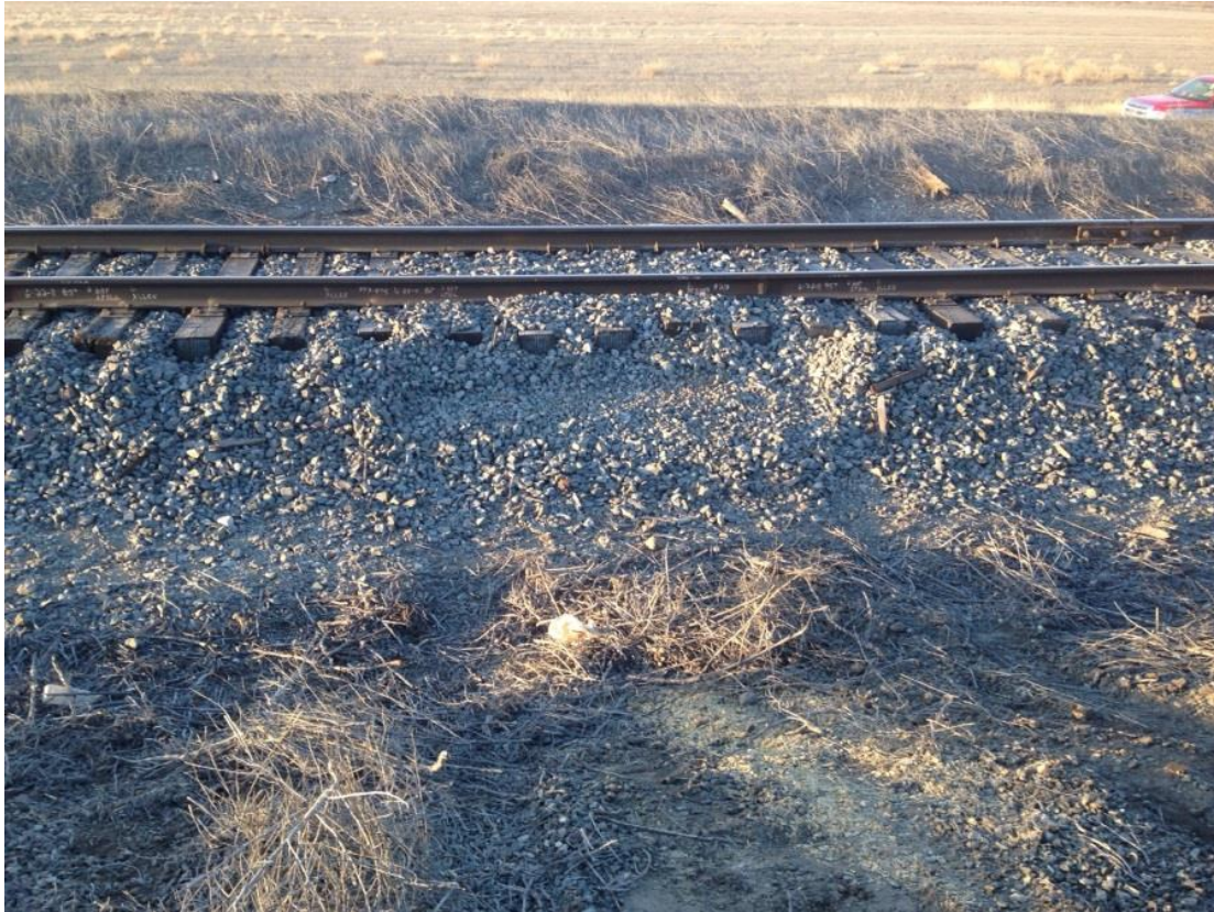
Figure 6. This is a view looking south at the track structure. Notice the disrupted ballast shoulder section and track structure movement (see Figure 3 for different perspective).
