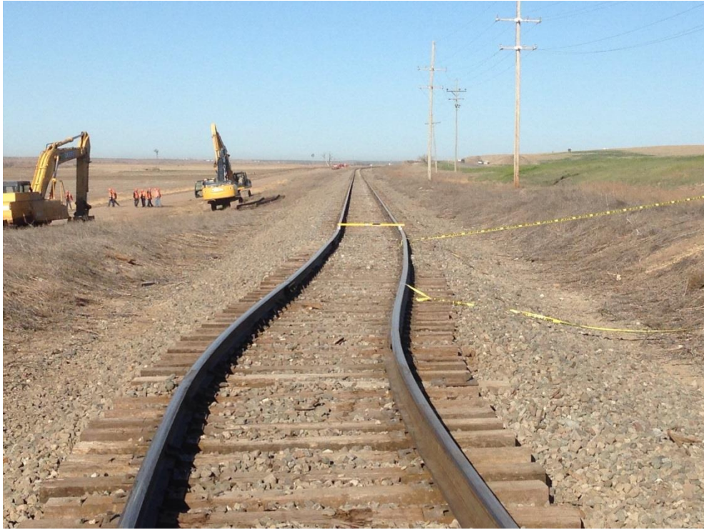
Figure 3. This is a view in daylight hours looking west from the point of derailment at the misalignment or lateral shift in its' "as found" condition after the train moved over the shifted track.
