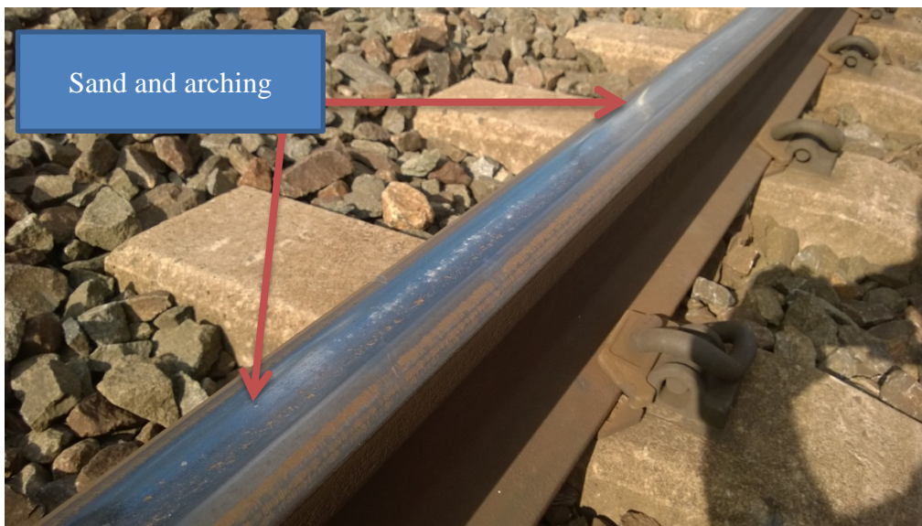
Figure 4-sand and arching on inside curve rail - west of POD
