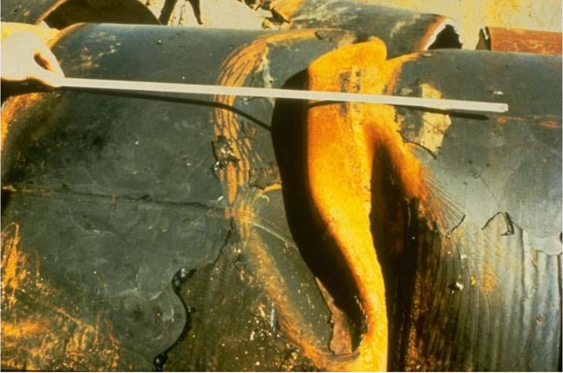
Figure 7. Wrinkled Pipeline Failed in Compression
