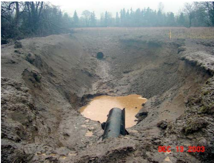
Figure 4. Crater Resulting from Williams 26-inch Pipeline Explosion in Washington State, December 13, 2003. (Photo Credit - Washington Utilities and Transportation Commission)
