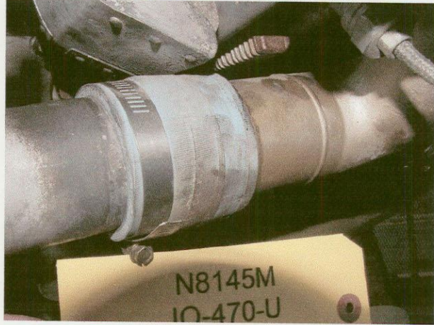
20. MISSING BAND CLAMP
