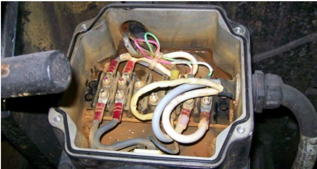
Exhibit IV-11: Water Intrusion into a Locomotive Junction Box
