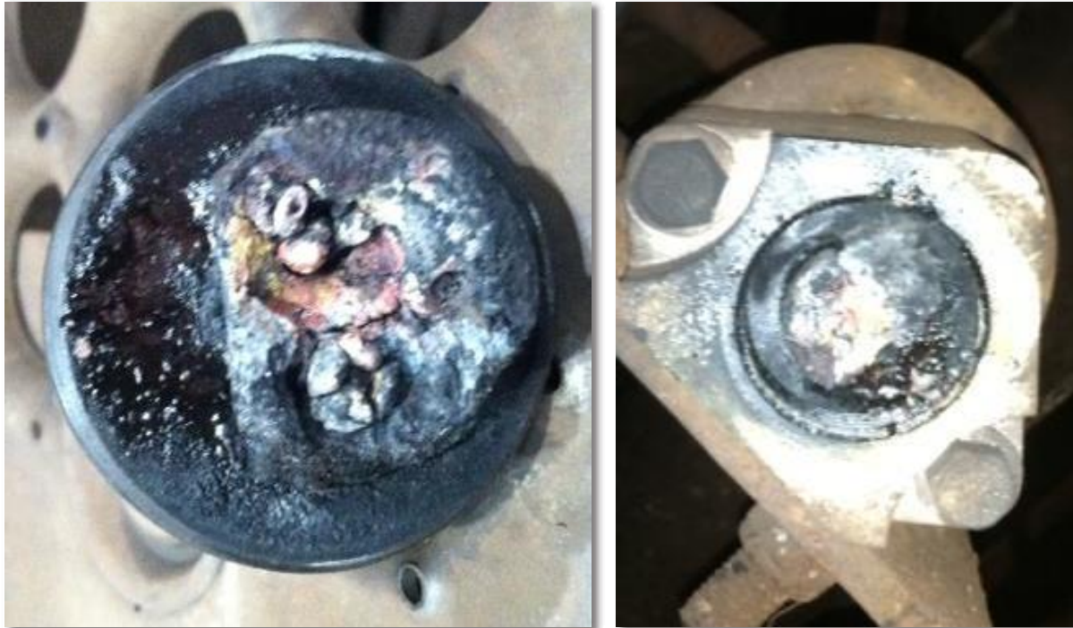
Exhibit IV-10: Water Intrusion into a Locomotive Junction Box Burned the Cable Connection to the Car Identification Module
