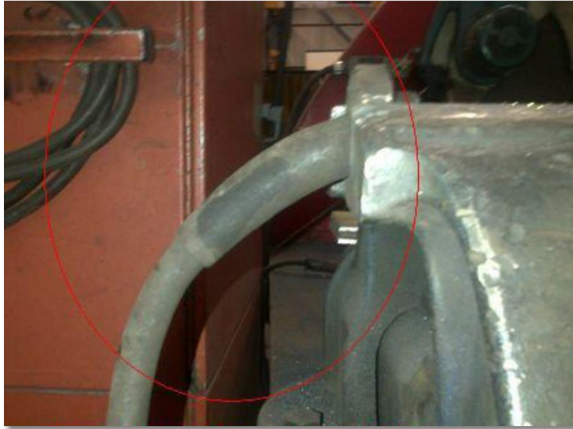
Excessive cable droop – likely will be bent
