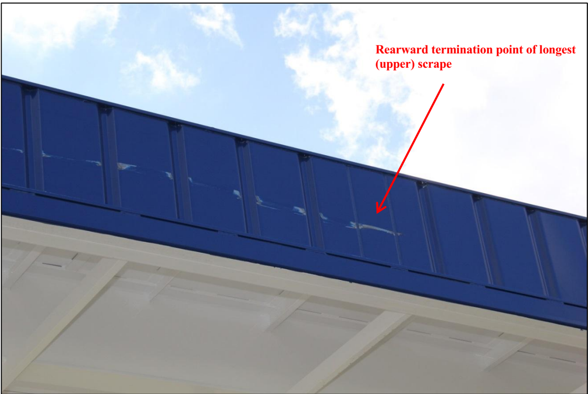
Figure 15: Rearward termination point of longest damage on left side of casing shed.
