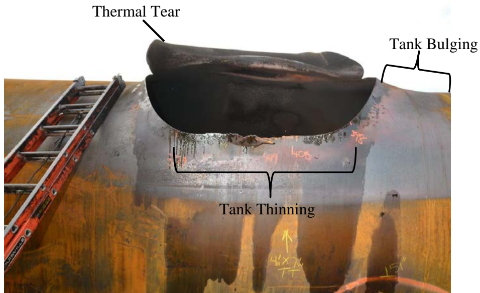
Figure 4: Tank car CBTX 741946 thermal shell tear surrounded by bulging and thinning shell.
