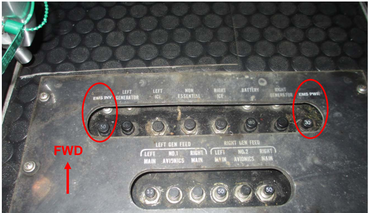
Figure 1 – Main bus tie circuit breaker panel from exemplar aircraft with additional STC circuit breakers identified (Note: accident aircraft STC C/B's were in a different position on the panel).
