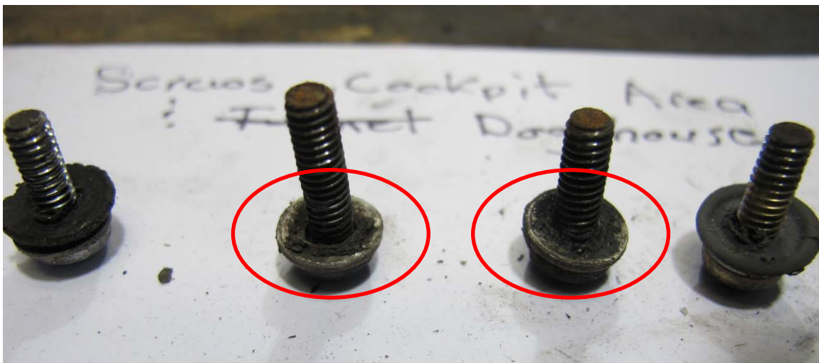
Figure 21 - Floor board attach hardware, screws missing rubber seals circled.
