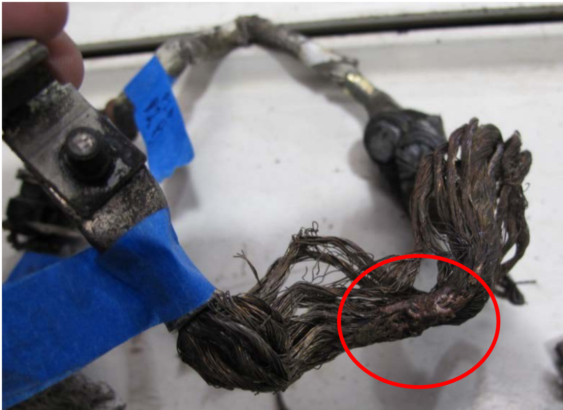
Figure 7 - Wire "P3H" with area of fused conductors highlighted.
