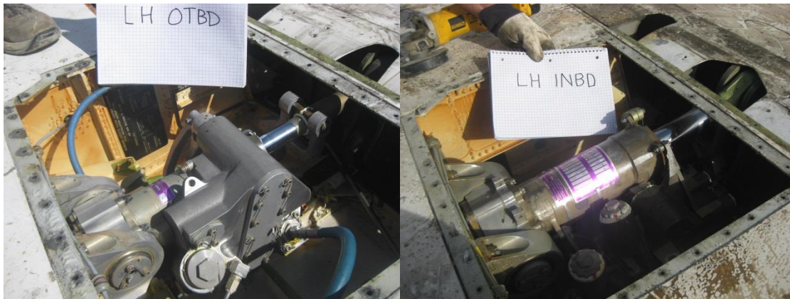
Figure 4 - Left Outboard PCU (Left) and Left Inboard PCU (Right), after access panels were removed.
