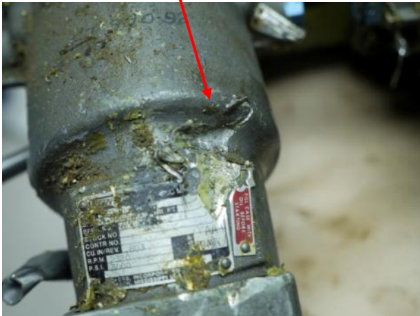
Figure 55: Left hand hydraulic motor damage
