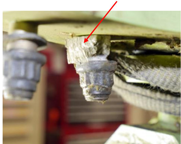
Figure 58: Piece of structure material
