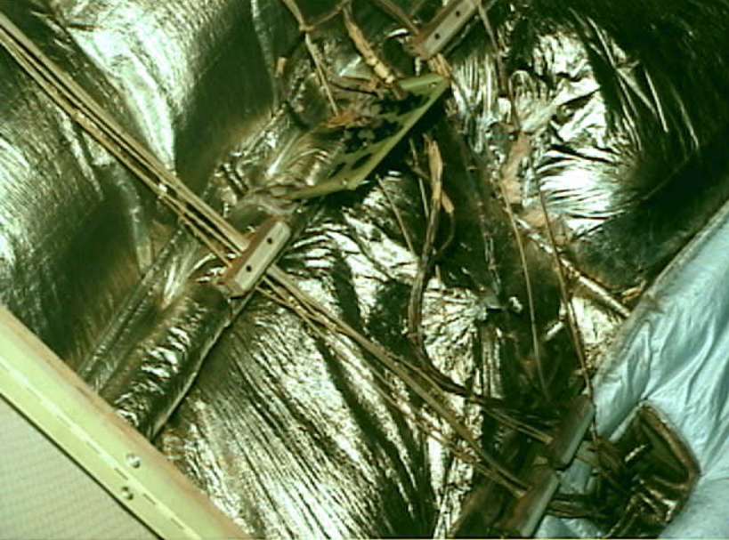
Systems 9 - Photo 9. Airplane 6. (1) B-747 Aft right upper fuselage insulation blankets stretch red & white wires not routed through clamps. (2) Sagging dark bundle contacts white bundle. (View is upward. Top of photo is upward).
