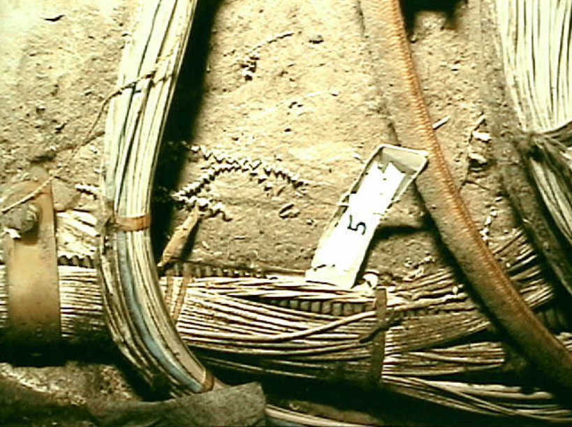
Systems 9 - Photo 7. Airplane 5. A-300 Electrical compartment beneath cockpit. Drill shavings shown on wires and shaving are between cable and wires. Loose string, wire chafe, and lint are visible. (Left edge of photo
