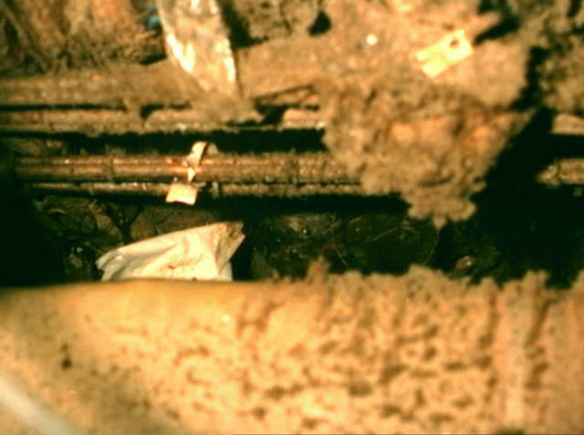
Systems 9 - Photo 55 - L-1011 incident of March 17, 1991 (Rec. A-91-70). Bay behind burned area contains two inches of lint fallen over generator cables, plastic wrapper, nutplate, hydraulic "B-nut," foil between generator cables, hose clamp, and paper.
