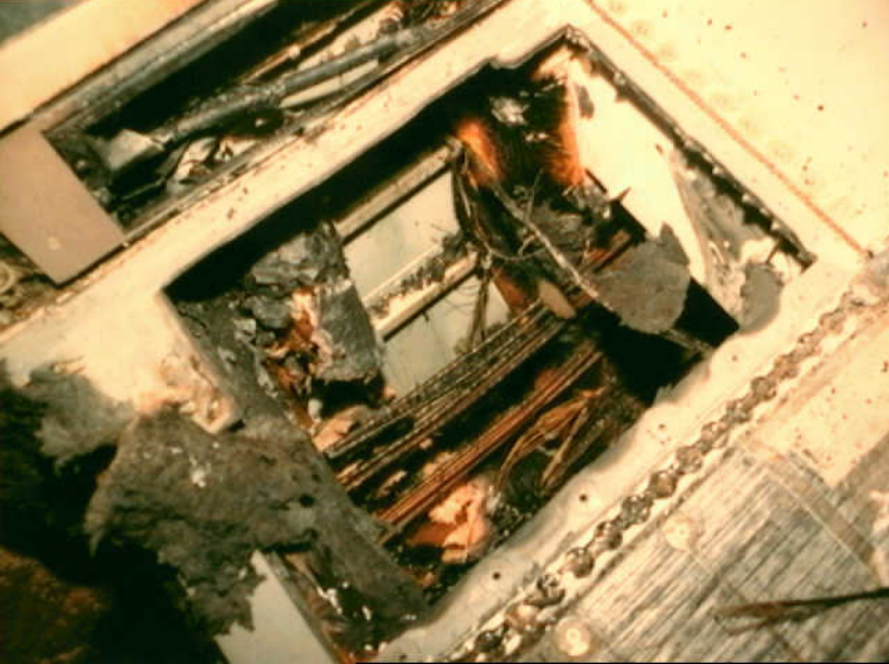
Systems 9 - Photo 54 - L-1011 incident of March 17, 1991 (Rec. A-91-70). Aft left fuselage beneath floor and seatrow 41, to left of C3 Cargo. Upper right corner of photograph is toward the nose of the airplane.
