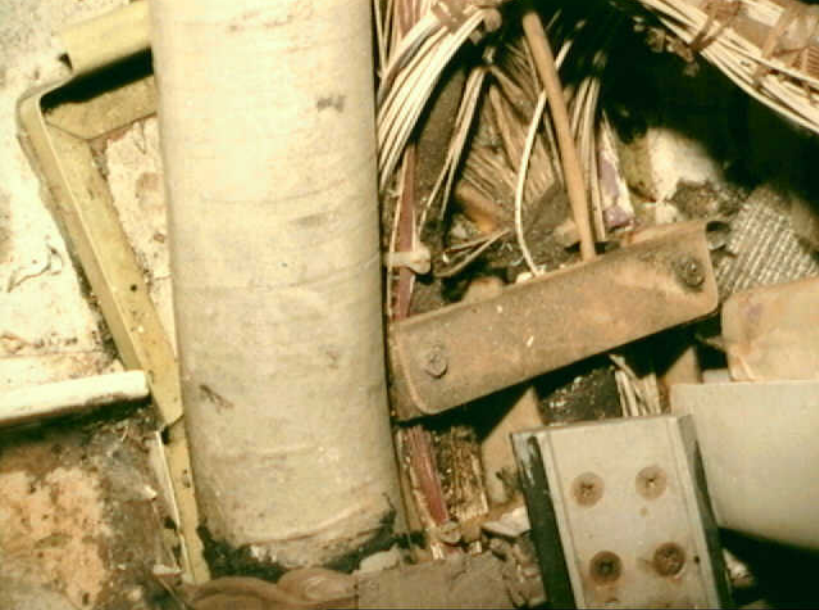
Systems 9 - Photo 49. (Feb. 21-25, 1998) B-747 W985 and other wire installations at forward corner of cockpit emergency escape (right) door. Visible ae trash, metal shavings, dirt, and flud stains. (View is down. Outboard is to right. Photo top is fwd.
