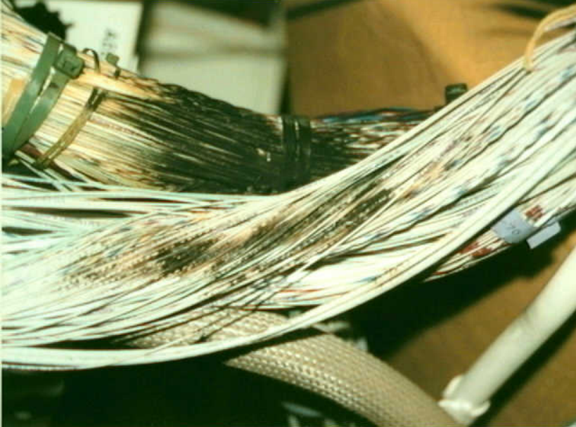
Systems 9 - Photo 43. Airplane 19. B-767 wires within the woven (Varglas) sleeve that the burned wires laid against. The wire insulation is bubbled and blackened.
