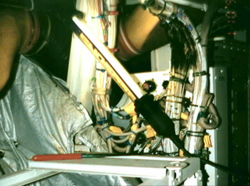
Systems 9 - Photo 41. Airplane 19. B767 burned wires seen after chiller removed from the rack over the oxygen tank. The edge of the chiller was near the burned area, damaged wire insulation was found on unburned wires, and foam on chiller burned.
