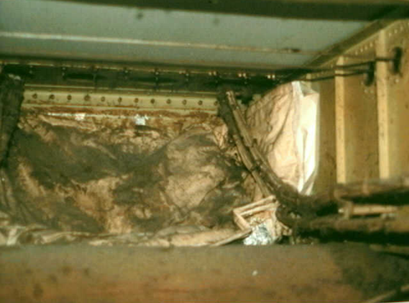
Systems 9 - Photo 40. Airplane 18. B-747 wire bundles containing CWT FQIS W480 along aft side of the station 920 floor beam. Lint visible on thermal insulation.
