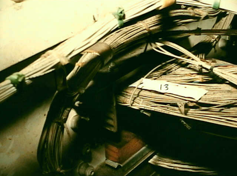
Systems 9 - Photo 30. Airplane 13. B-747 station 400 (right) opening with clamp loosened for photo. Insulation of adjacent wire chafed off at nylon edge of clamp. Also visible are a mixture of new and old wire and drill shavings.
