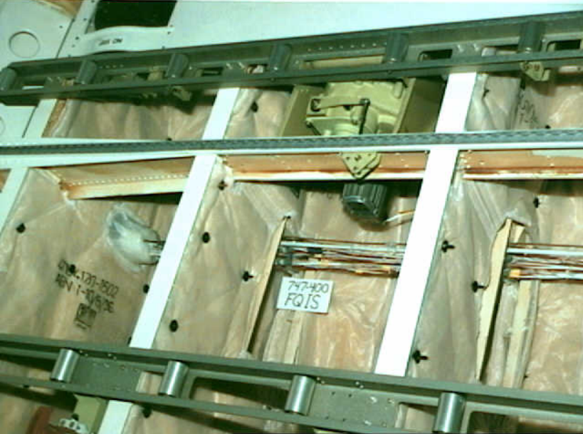
Systems 9 - Photo 3. Airplane 3. Exposure of fuel quantity and fire system wire bundles in B-747-400 forward cargo compartment, beneath aft cargo motor. No covers have been removed. (View is down. Right edge is forward).
