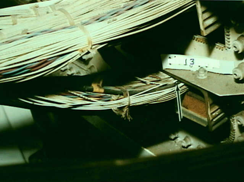
Systems 9 - Photo 29. Airplane 13. B-747 station 400 (left) opening with clamp loosened for photo. Arrow points to hole worn through black woven sleeve on wires. Wire in sleeve was damaged. Loose string ties visible. Clamp above is missing retainer.
