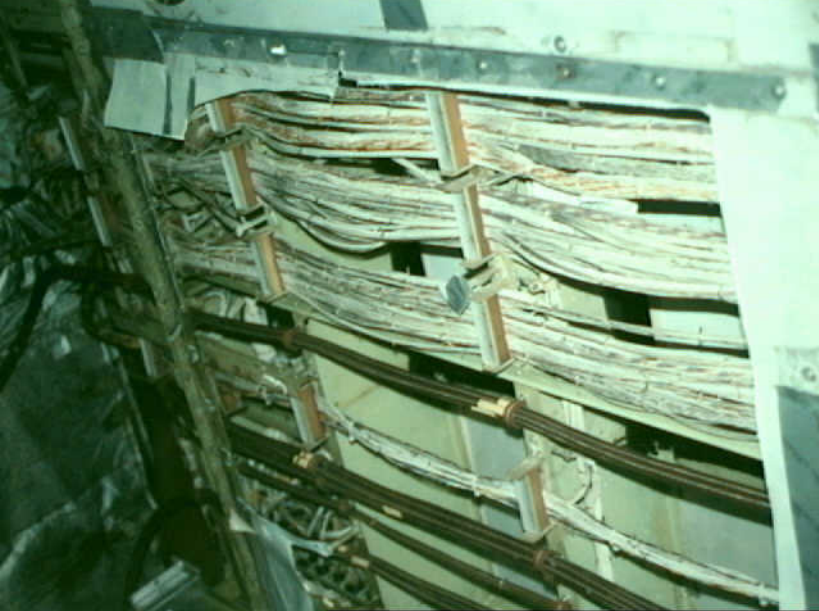
Systems 9 - Photo 27. Airplane 12. B-747 over forward cargo compartment with left side of the forward spar visible. The cargo compartment ceiling liner has been removed. (View is aft-right and forward is to right of
