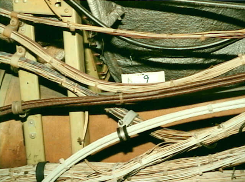
Systems 9 - Photo 19. Airplane 9. B-747 upper deck. CWT FQIS wires in bundle W480 sag and rub on galley power cable. Also visible are mixture of clamp types, mixture of wire types, broken clamp retainer at lower left and sags in upper bundles.
