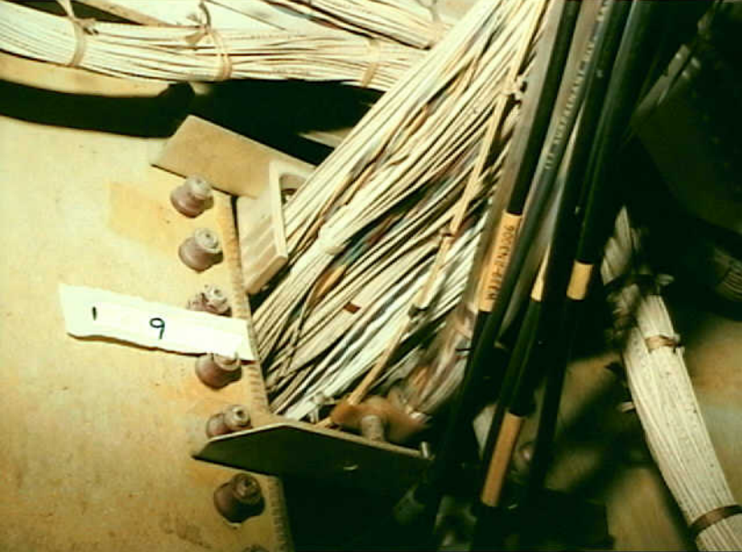
Systems 9 - Photo 17. Airplane 9. B-747 Raceway clamp at STAT 400 opening has no retainer. Pressing upward on wires revealed that the quantity of wires prevented installation of a retainer. Mixed wire types and fresh white wire insulation is visible.
