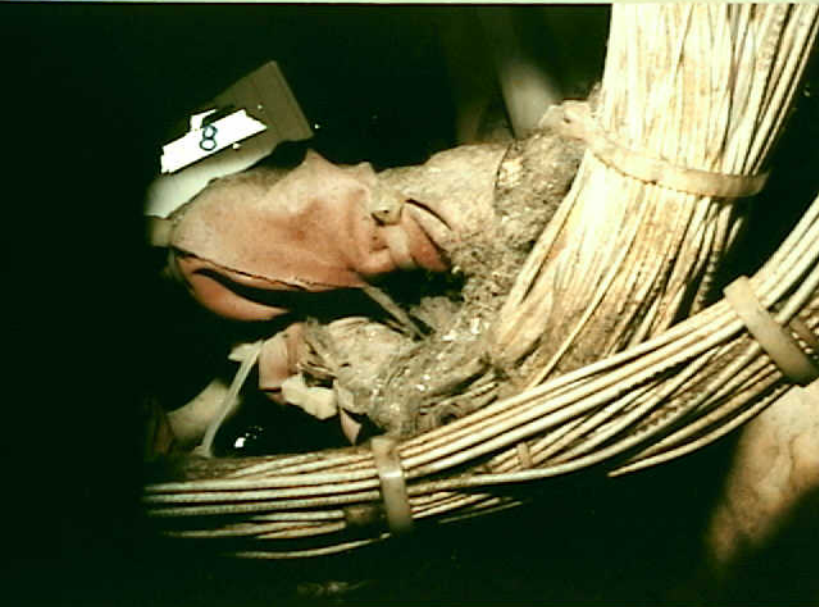
Systems 9 - Photo 15. Airplane 8. DC-9-30 Lint and metal shavings in electrical equipment center, behind left avionics racks.
