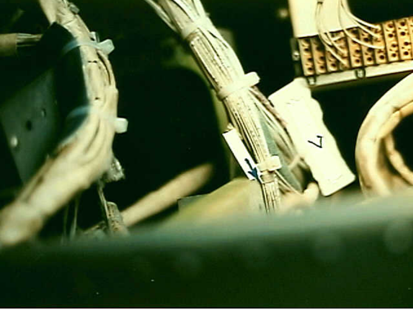
Systems 9 - Photo 10. Airplane 7. Arrow points to wire rub on structure behind B-747 flight engineer panel. Paint rubbed off metal to right. Lighting is sunlight from aft right cockpit window. (Right edge of photo is up)
