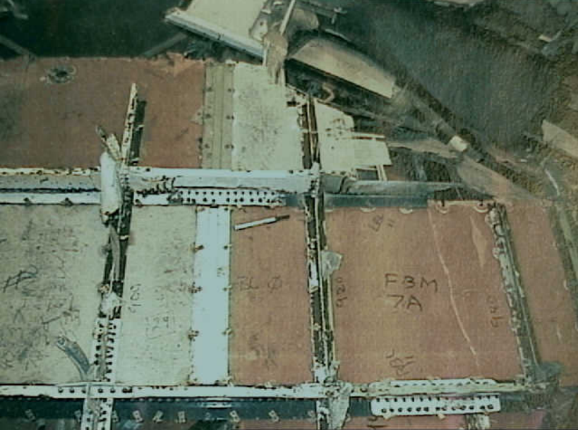
Systems 9 - Fuel Quantity Indication System - Photo 9. Structure repairs from bottom of main deck cabin floor. Location is ahead of forward spar. Repairs are to left and right of the airplane centerline, which is marked "BL 0." Left edge of photo is forwa
