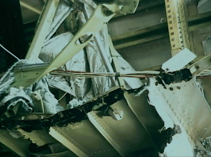
Systems 9 - Fuel Quantity Indication System - Photo 43. W480 (& other) bundles from upper deck at about station 53-560.
