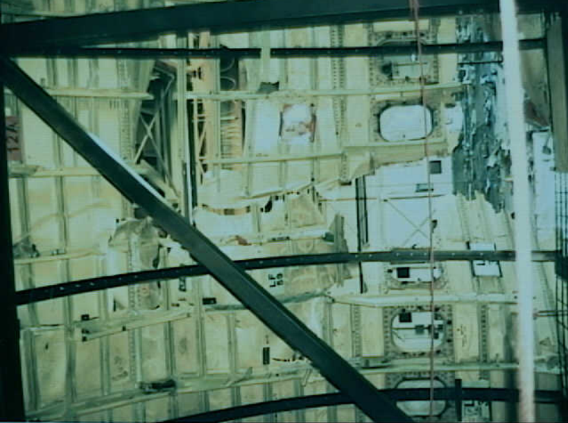
Systems 9 - Fuel Quantity Indication System - Photo 38. Left side of fuselage at station 920 (wire is missing near opening).
