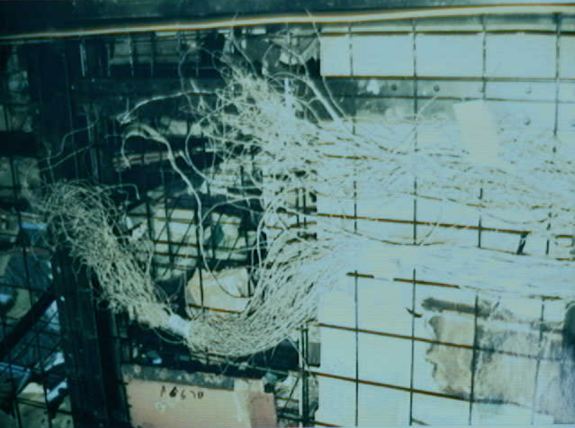
Systems 9 - Fuel Quantity Indication System - Photo 36. W480 (& other) bundles from forward of CWT, between stations 1030 to forward end of bundles from about station 95.5. Generator cables visible beneath floor level.
