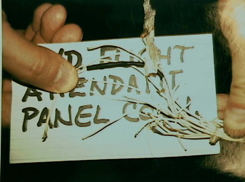
Systems 9 - Fuel Quantity Indication System - Photo 29. Repair found to wiring behind upper deck flight attendant control panel.
