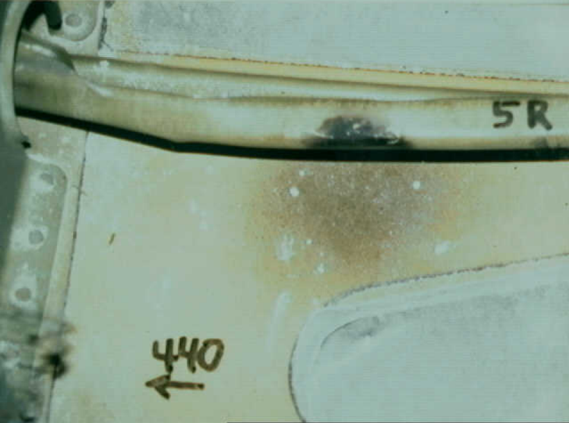
Systems 9 - Fuel Quantity Indication System - Photo 26. Darkened area on stringer 5 (right), near station 440 frame.
