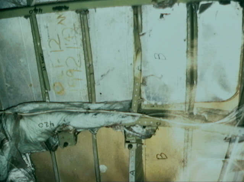
Systems 9 - Fuel Quantity Indication System - Photo 25. Sheetmetal repair and hand-written "OCT. 12 1992 1:42AM". Also visible are different shades of green and white paint.
