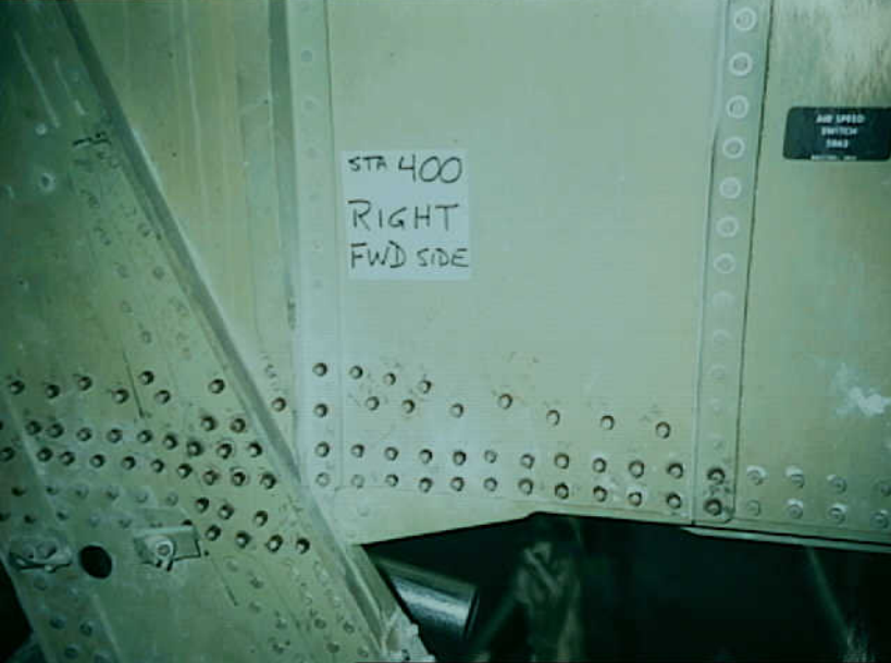
Systems 9 - Fuel Quantity Indication System - Photo 17. Repair found in frame at station 400 (right), beneath route of W350 and W1360 wire bundles.
