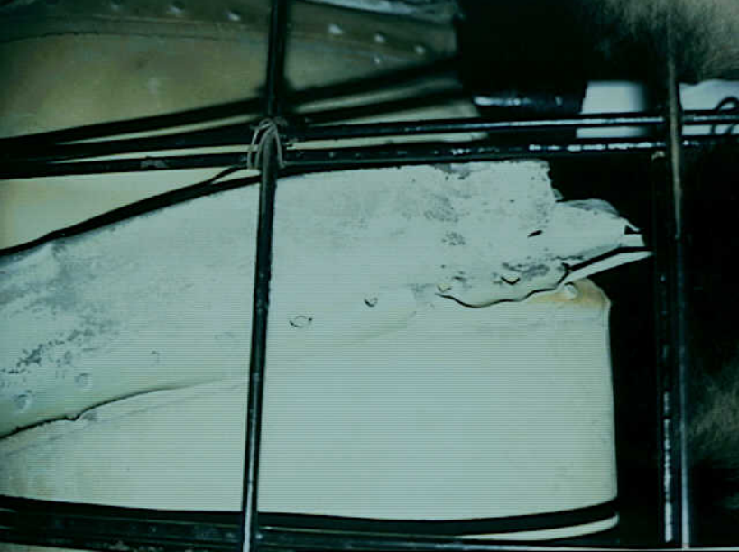
Systems 9 - Fuel Quantity Indication System - Photo 16. Different colors of paint and paint overspray on stringer at station 360, along route of W350 and W1360 bundles.
