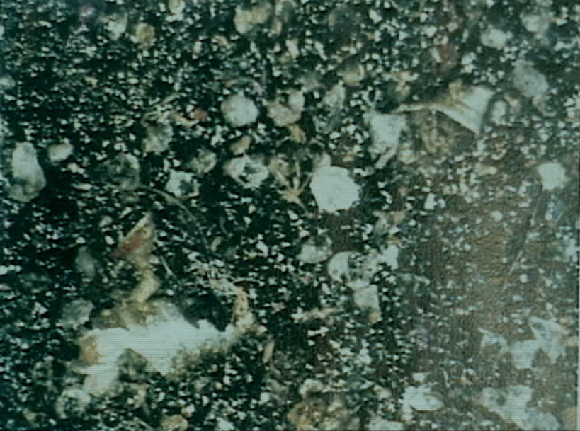
Systems 9 - Fuel Quantity Indication System - Photo 12. Drill shavings visible in sealant at bottom of STA 920 floorbeam. (Digital image)
