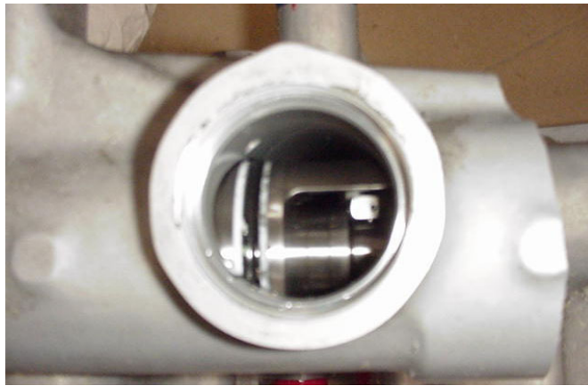
Figure 6 – Interior of Manifold
