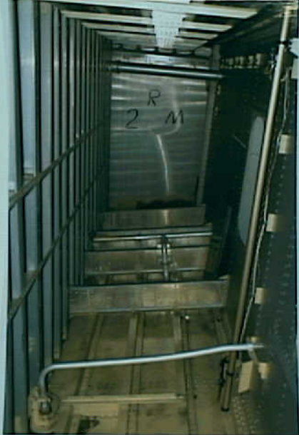
Systems 9 - Exhibit No. 9E - Photo No. 7 - In CWT, looking across between spanwise 2 and mid-spar. Shows fuel probe, compensator, and scavenge pick-up. (N93105). ATA 28-41-01.
