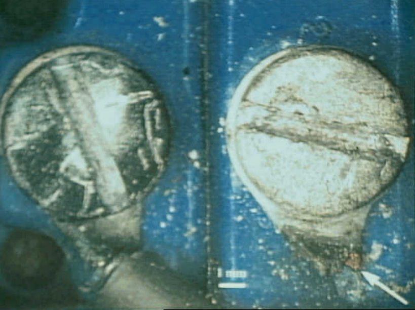
Systems 9 - Exhibit No. 9B - Photo 5. Figure 5a. Left jettison switch screw terminals exhibiting corrosion from salt water exposure. Note the exposed copper from the solder lug (arrow).
