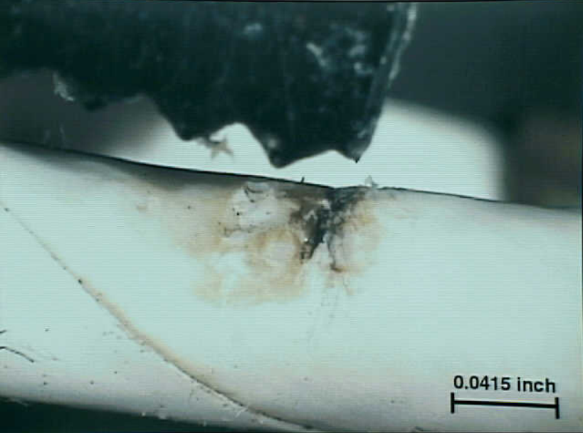
Systems 9 - Exhibit No. 9B - Photo 33. Figure 33g. Damage to PTFE insulation caused by serrated surface and clamping pressure.
