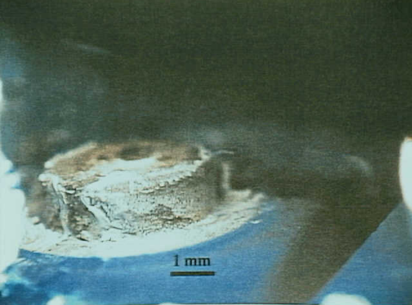
Systems 9 - Exhibit No. 9B - Photo 24. Figure 24a. Normally open stationary contact surface of the right jettison switch exhibiting salt water-like residues.
